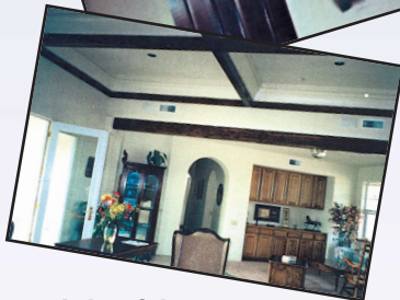
The remainder of the house was undamaged.
