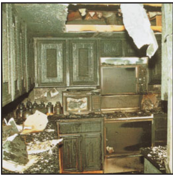
Kitchen fire without fire sprinklers
